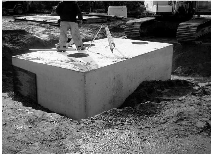
The swirl reactor being installed at Mettatuxet Beach. The openings on the top will allow periodic inspection and removal of accumulated sediment
