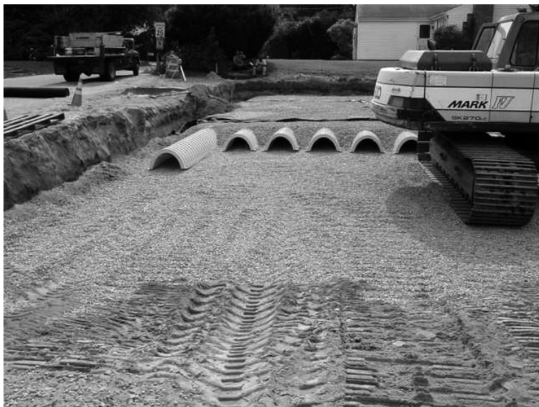
Installation of the Cultech component of the Mettatuxet treatment system. The perforated pipes are only partially in place and being buried in fine gravel. The entire thing is now hidden below the parking lot.
